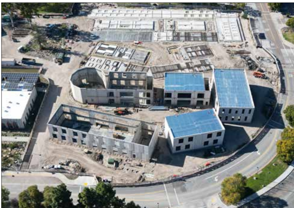
Buildings are being developed and construction is ongoing at Southwestern College, where the school is currently putting in a Student Union Complex , an Instructional Complex and a Landscape Nursery Technology space . Photo courtesy Southwestern College
